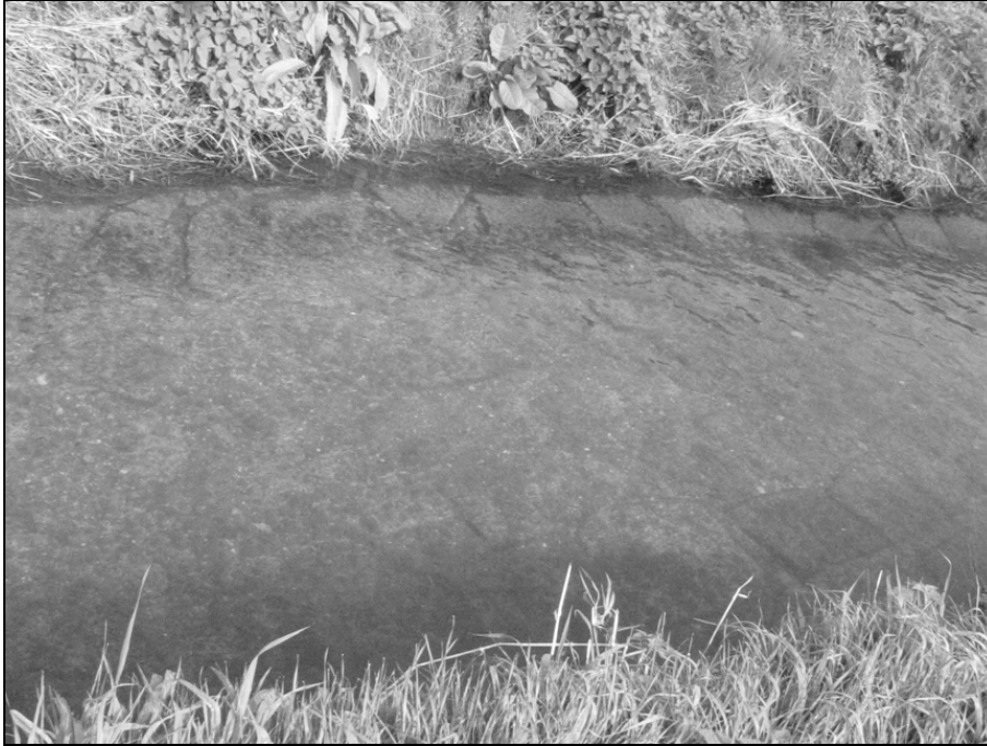
Figure 6: The paved bed of the “Urfahrner Sammelgerinne” in Linz before the restoration.
